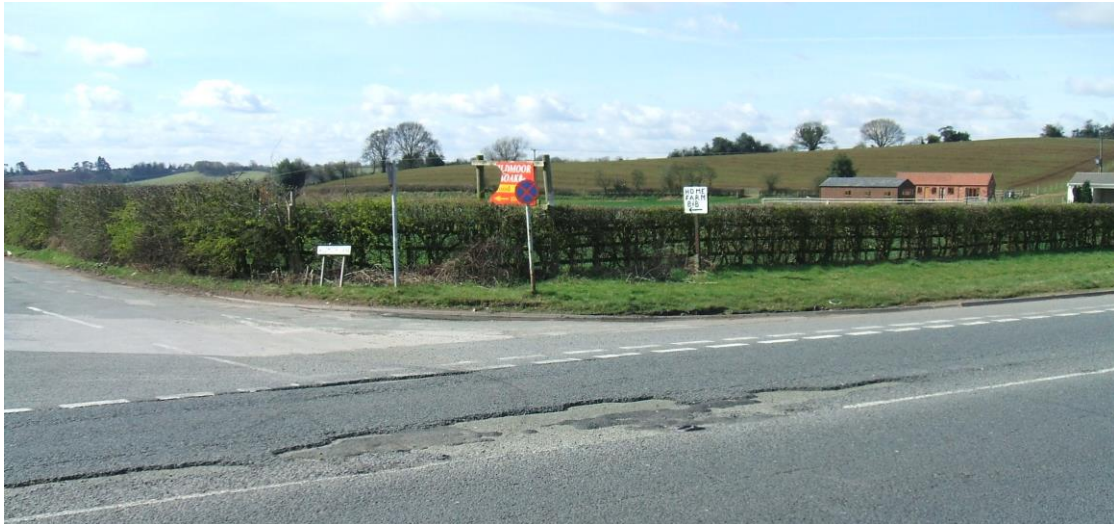
Example of abrupt level difference in carriageway
