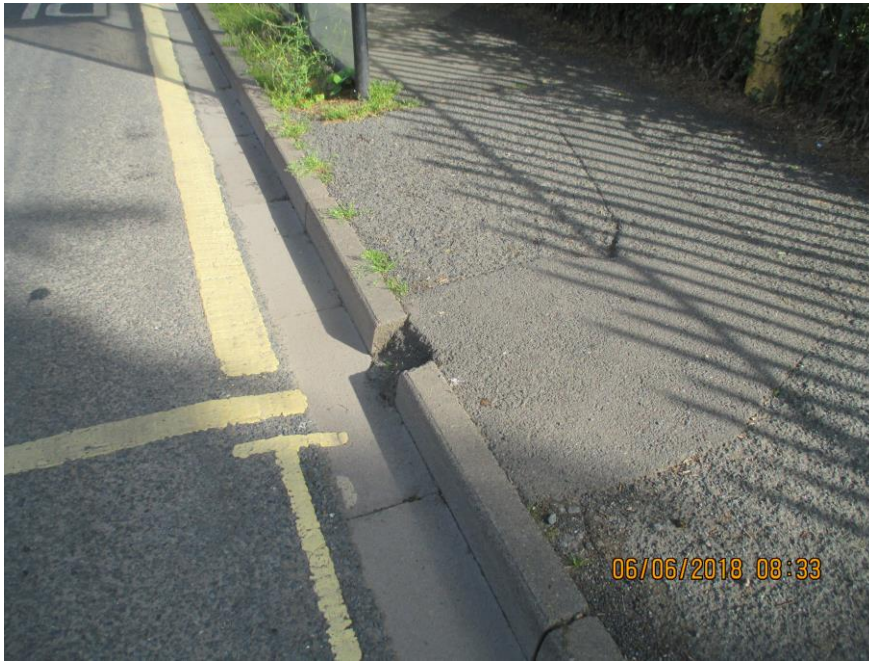
Example of gap in kerb line
