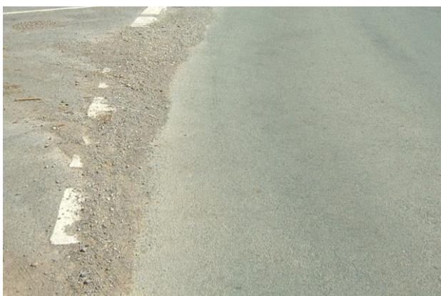
Example of loose gravel at road junction.
