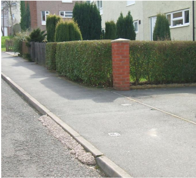
Example of an Illegal concrete ramp in channel.
