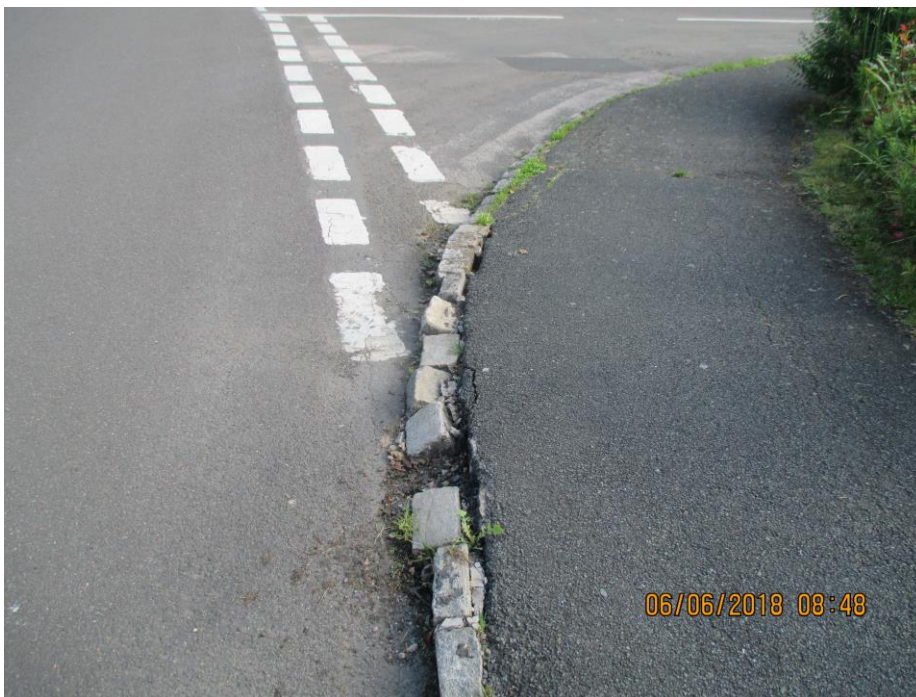
Example of damage granite set kerbs
